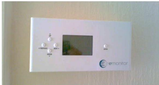
Energy Billing call this an “EE Monitor”
